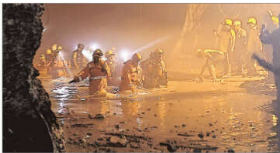
Water and debris entered a tunnel under construction at a hydroelectric project site in Chamoli, Uttarakhand, on Thursday
