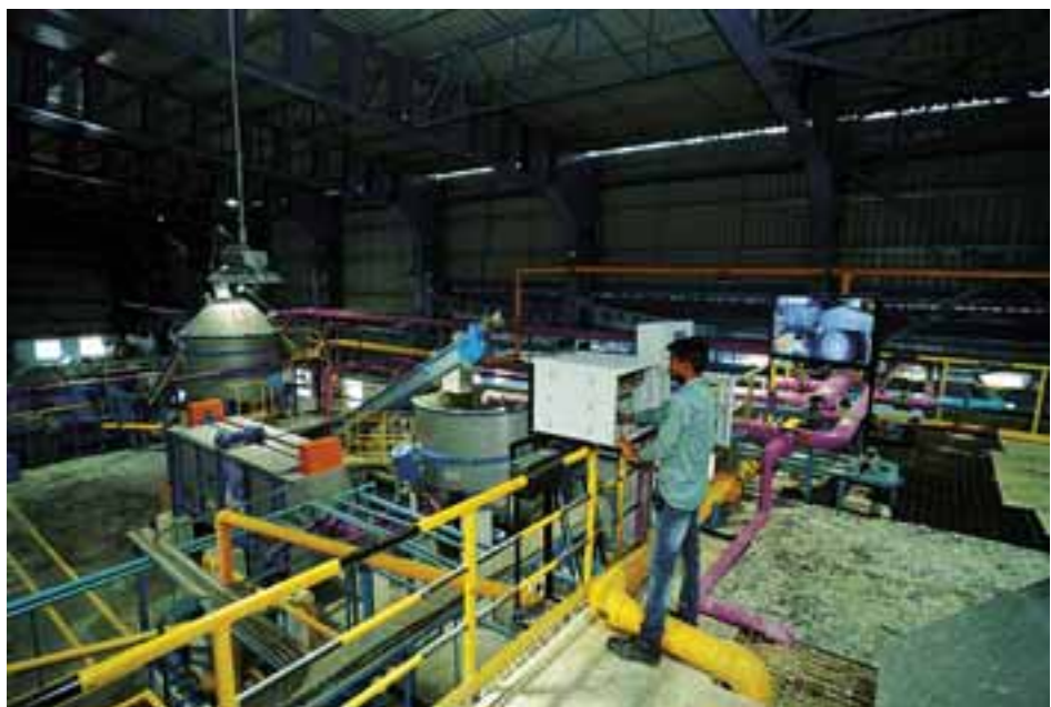
The UFlex recycling plant for liquid packaging in Gwalior, Madhya Pradesh
