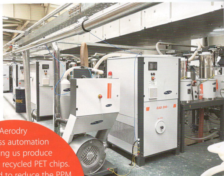
PET flakes crystalliser and dehumidifying drying systems.
